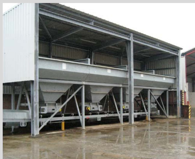
Day bins for filling with loader.
