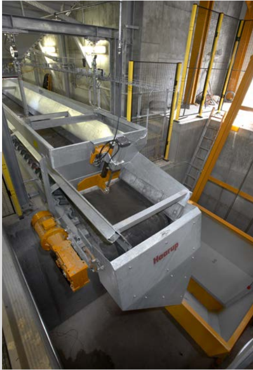
Weigh belt and hoist.
