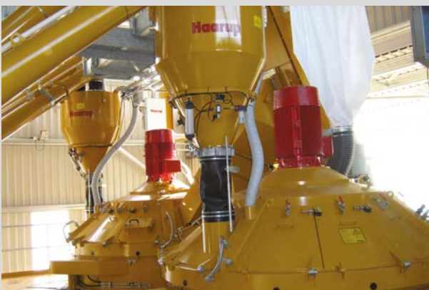
Cement weigh hoppers suspended in electronic load cells.
