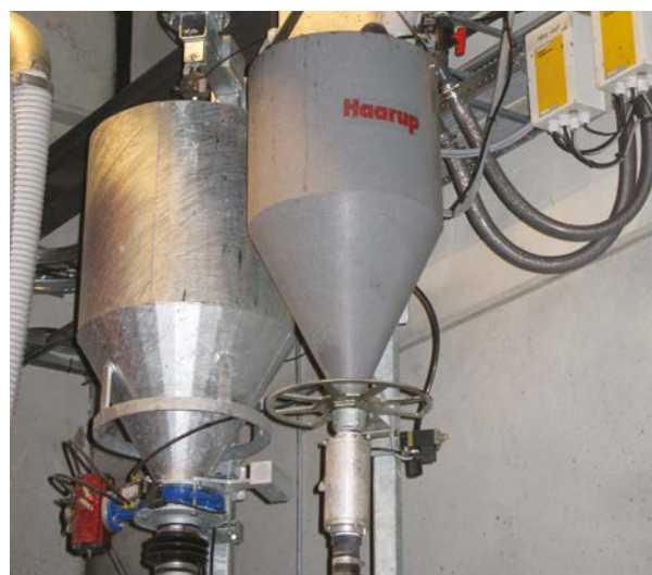
Slurry-colour and water weigh hopper with inlet and outlet valves.
