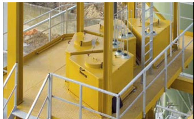
Four 1500 litres dry colour hoppers on a platform.
