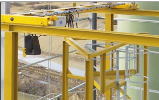
Gantry crane for Big Bags intended for charging into colour hoppers.
